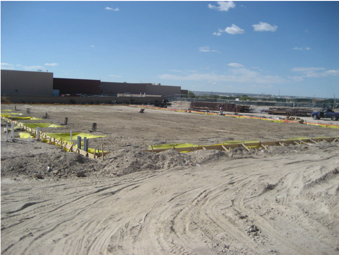
The start of rebar- which will help form and hold the slab
